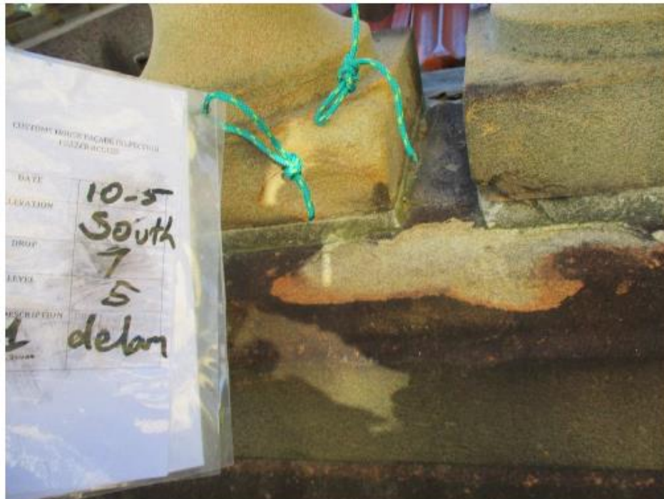
Level 5: sandstone deterioration at base of balustrades
