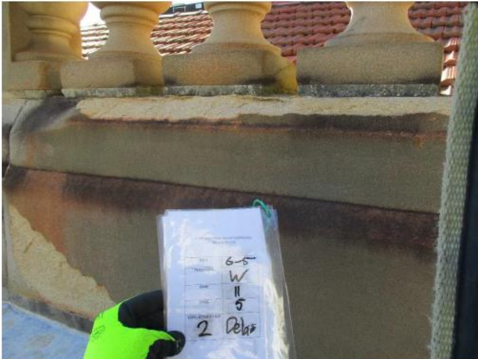
Level 5: deterioration at base of sandstone balustrades
