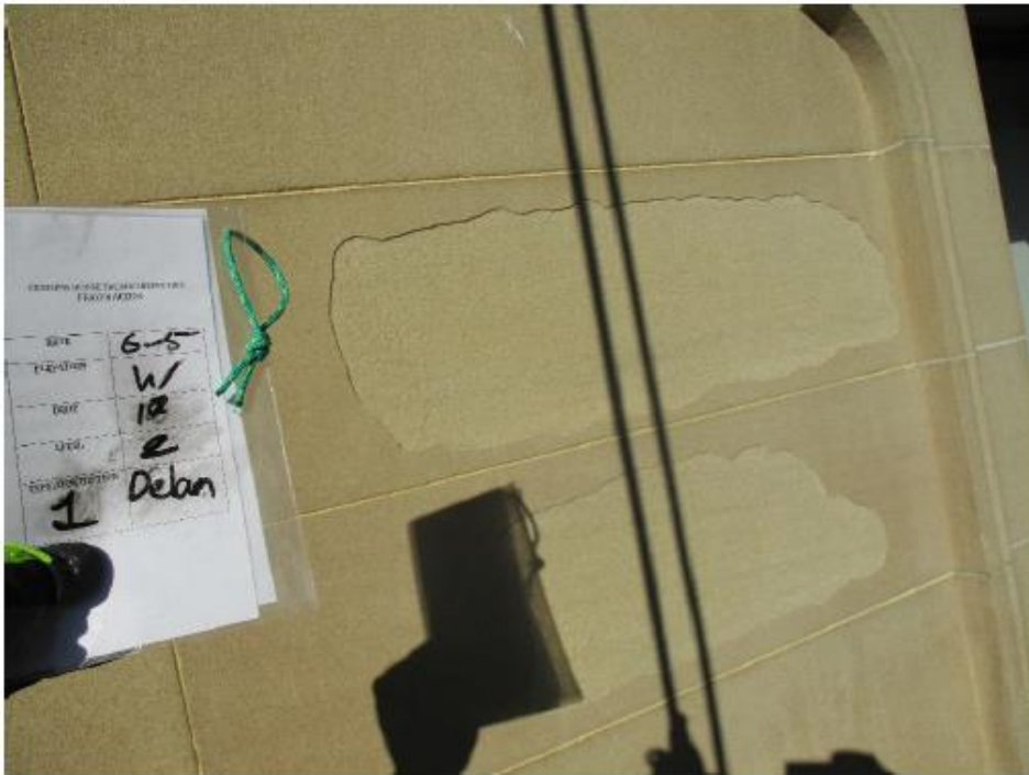
Level 2: weathering of sandstone wall
