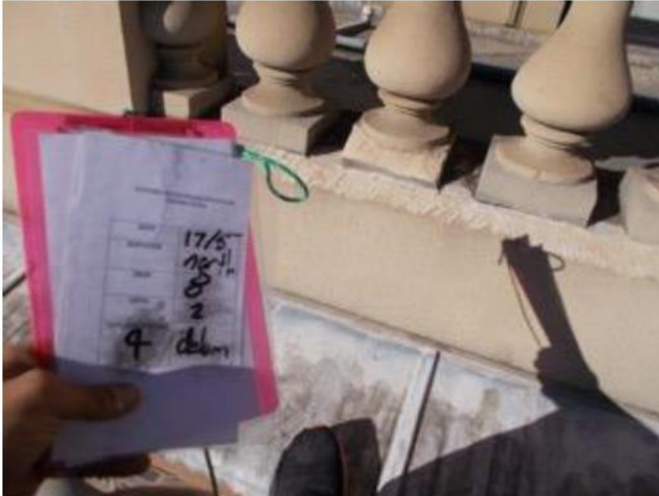
Level 2: deterioration at base of sandstone balustrade
